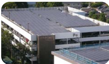
Tokyo Electron Yamanashi's PV power generation system
