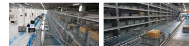
Tokyo Electron Miyagi JIT Supply Center (Automated Warehouse)
