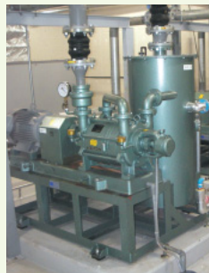
Vacuum pump that uses recirculated water
