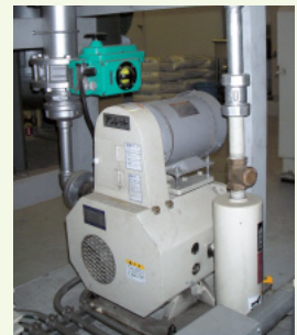
Vacuum pump that does not use water
