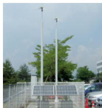
Hybrid power generation system
