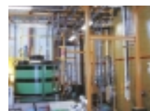
Wastewater treatment facilities
